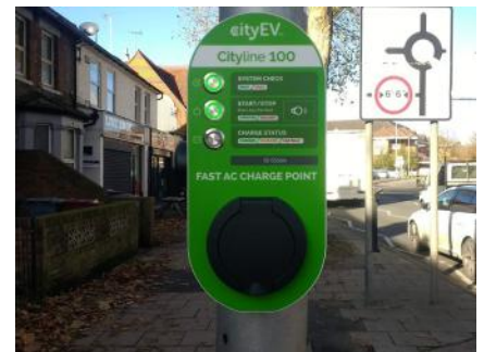
READY TO GO: a new charging point in Caversham Road
